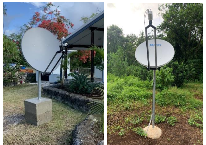
Newly install satellite dish after TC Harold
